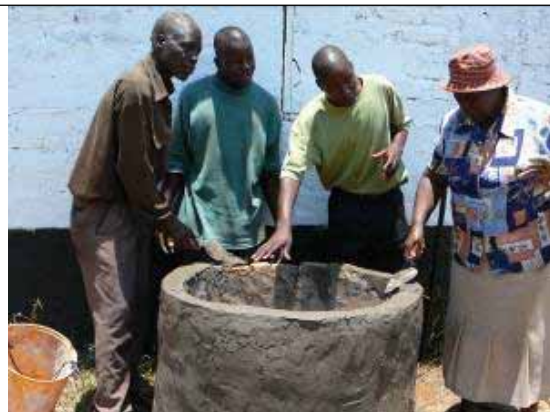
Finish inside and outside and as last part bottom and outlet pipe
